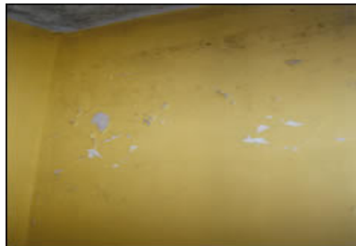
Typical mould damp damage caused by poor ventilation
